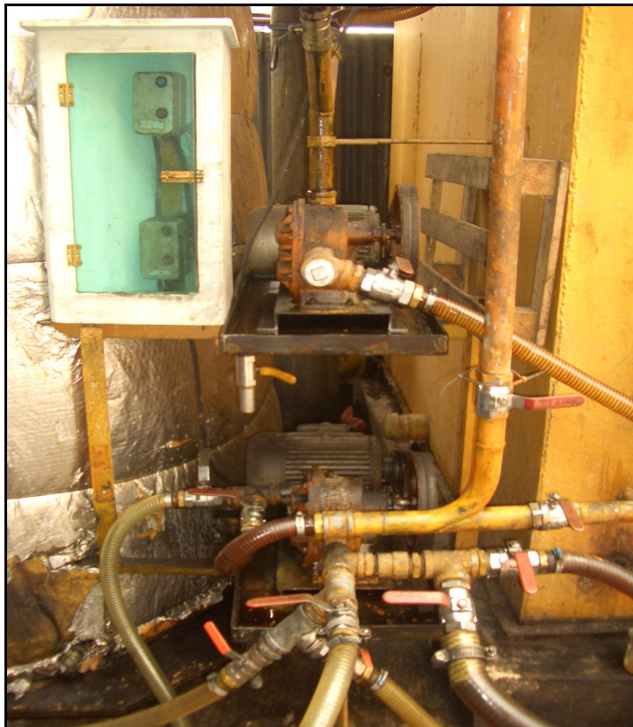
Photograph 4-1 Drip trap to Collect and Recycle Oil ( at the pilot plant )
